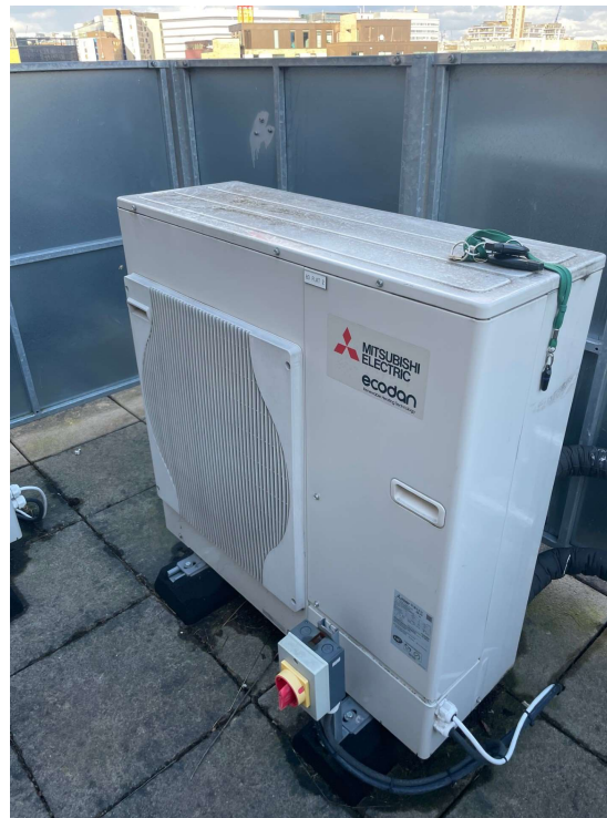
Air Source Heat Pump for a 2 bedroom flat.
